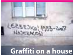
Graffiti on a house
